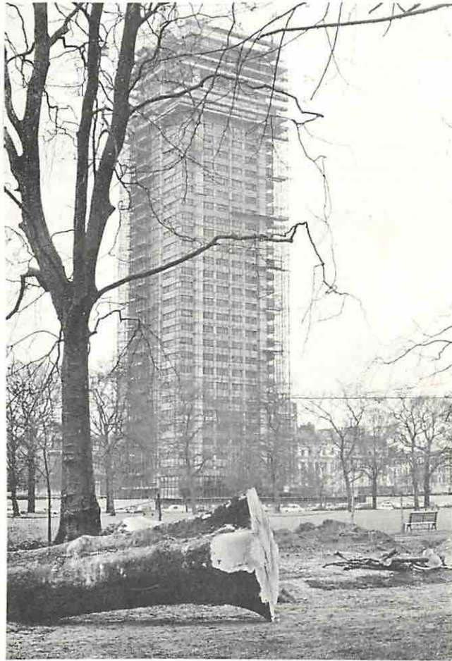
The new Knightsbridge Barracks under construction at the Southern edge of Hyde Park
